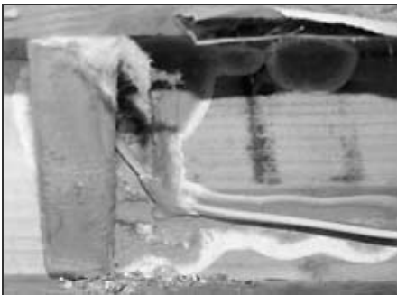
Figure 4 (continued). Wood Rot — Poria
